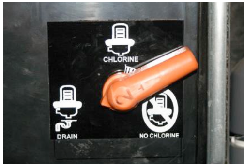
Figure 38 – Drain the Chlorinator
