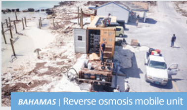
BAHAMAS | Reverse osmosis mobile unit
